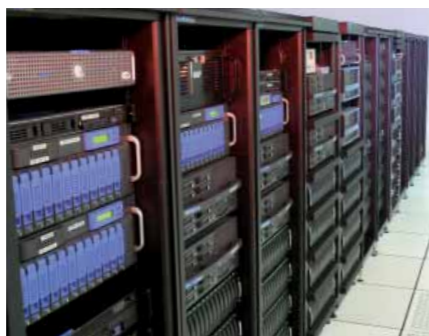
Data Centre Management and infrastructure
