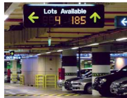
Parking Guidance System
