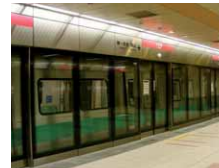
Platform Screen Doors
